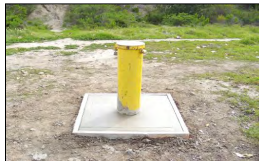
Monument Well Cover and Concrete Pad
