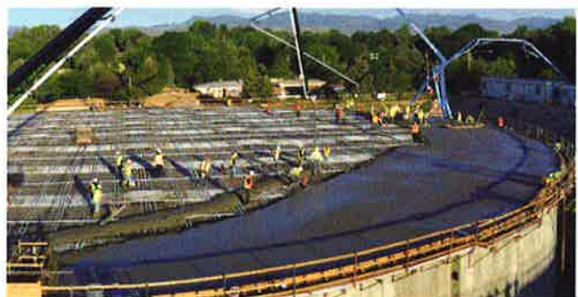
10 MG concrete storage tank in Wheat Ridge, Colorado.
